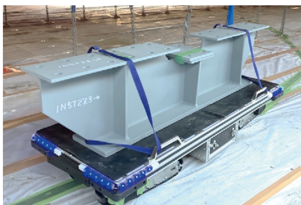
AGV for transporting materials
