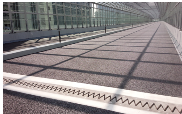
KMA Joint on the Kachidoki Flyover
